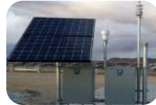
PV Weather Monitoring
