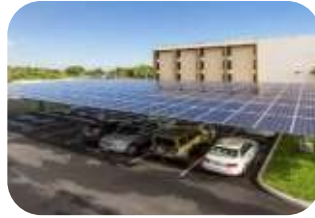
PV Parking Canopies
